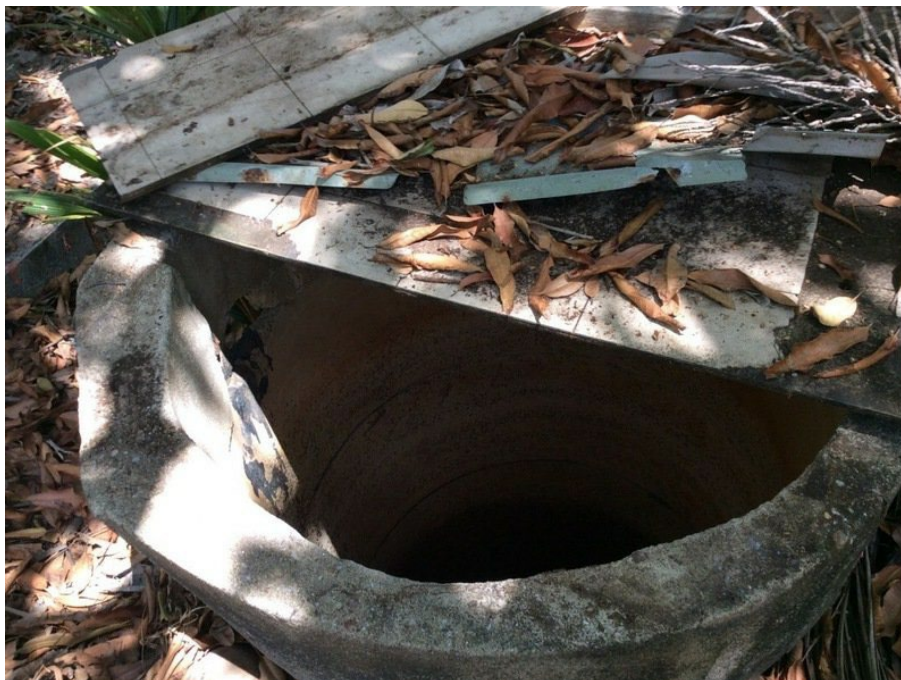
Figure 21: St Paul's Kurrsarr Well is a concrete lined circular well located adjacent to the community gardens. The well has a total depth of 2.22 m bgl.
