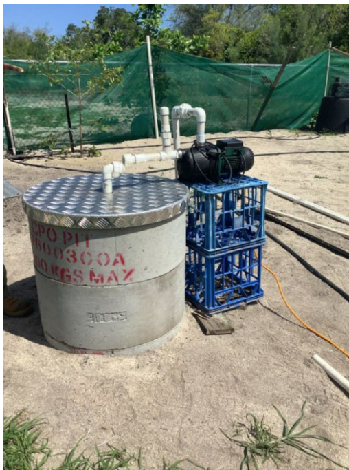
Figure 25: Thelma Billy Well is a concrete lined circular well located on Masig Island.
